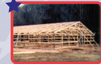
2" x 4" Roof Purlins spaced 24" apart, laid flat and overlapped approx. 1'. * Optional 2" x 6"
